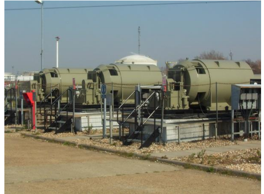
TOP: Aviation fuel refinery pumping station.
